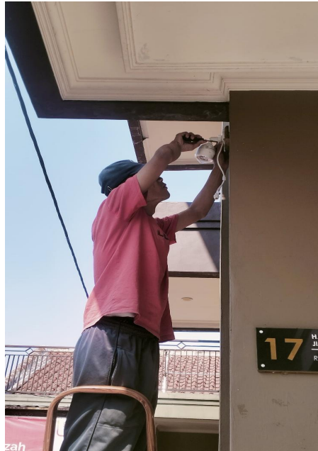
Figure 3. CCTV installation process carried out with local residents
