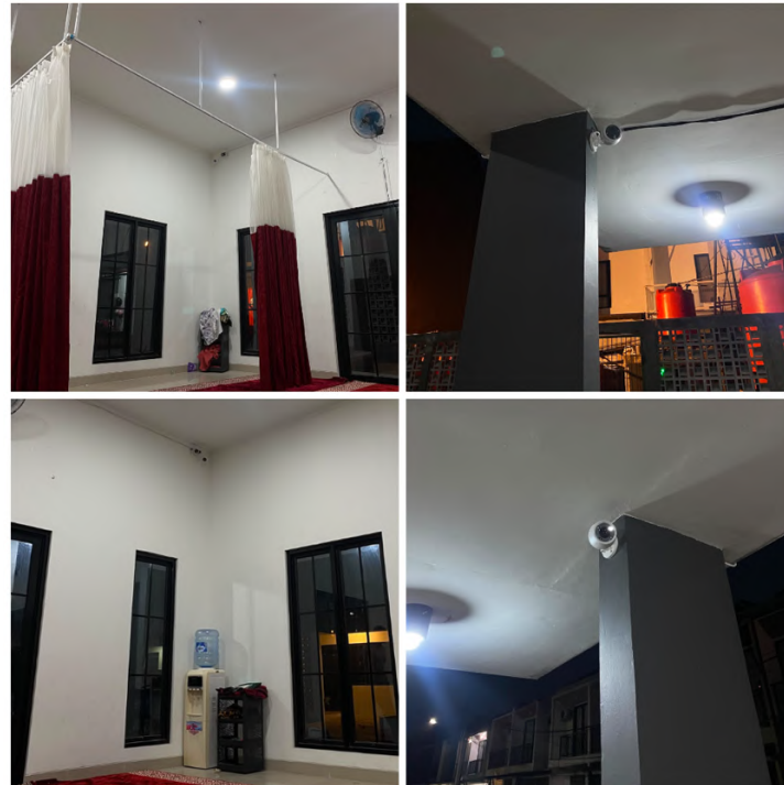
Figure 4. Implementation of CCTV outdoor and indoor according to camera placement plan
